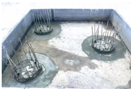
桩头部位渗漏
